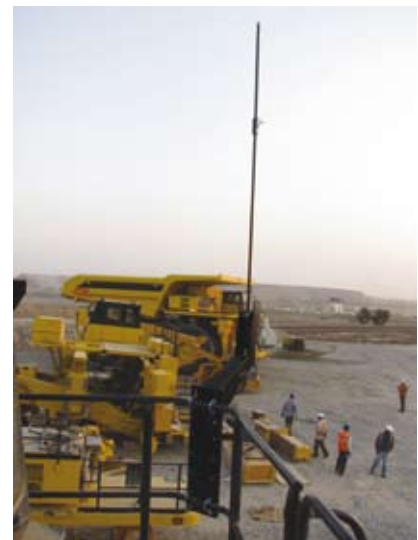
Figure 5. Komatsu 830Es under assembly at Hindustan Zinc's Rampura Agucha mine, with Modular® GPS antenna in the foreground.
